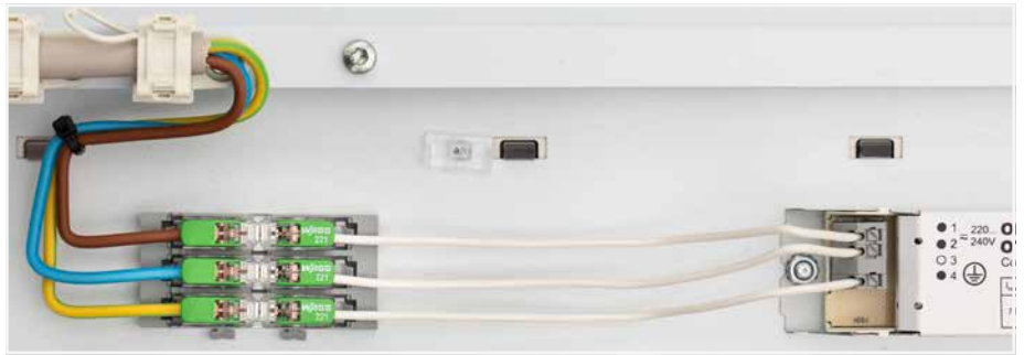
Wiring in the ceiling light.
