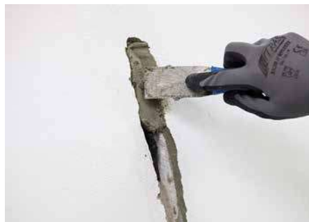
Close the damaged area discreetly.
