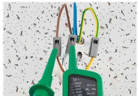
Testing via separate test ports.
