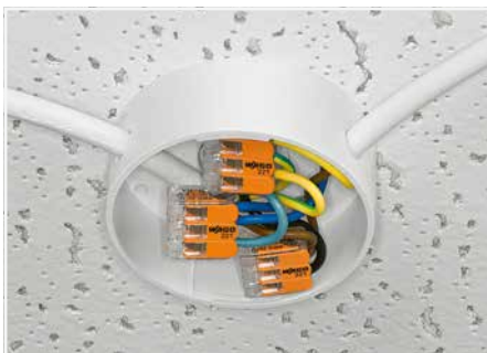
Lighting distribution in ceiling canopy
