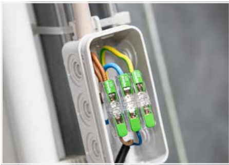
Wiring in the distribution box.
